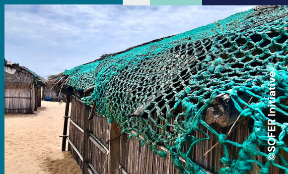
Figure 17: A repurposed fishing net being used to protect a thatched roof in a village in Nigeria.
