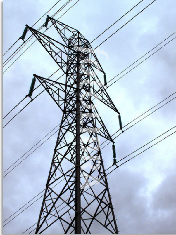
Figure 6-1: Typical Electrical Pylon
